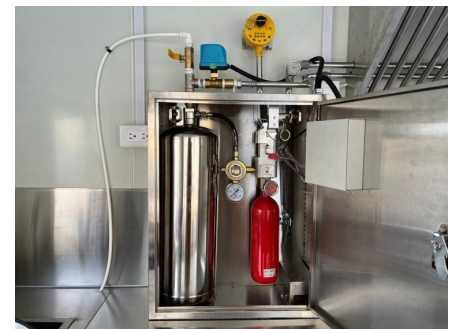
- Fire Suppression System -
